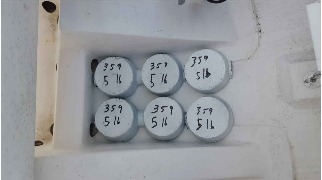
Starboard Battery box
