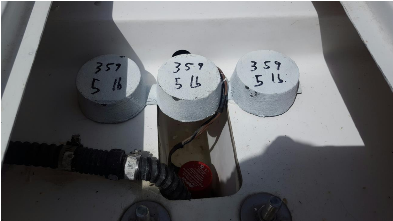
Forward Bilge at bilge pump sump
